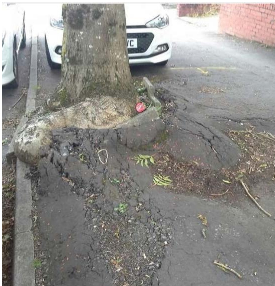
Example of Tree Root Damage
