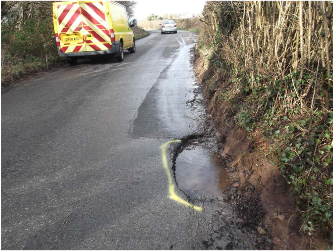
Example of Edge Deterioration
