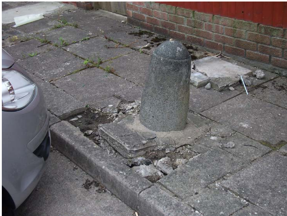
Example of Paving Defect
