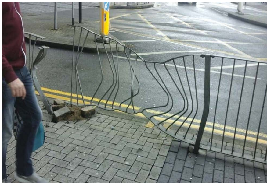
Damaged Pedestrian Barrier
