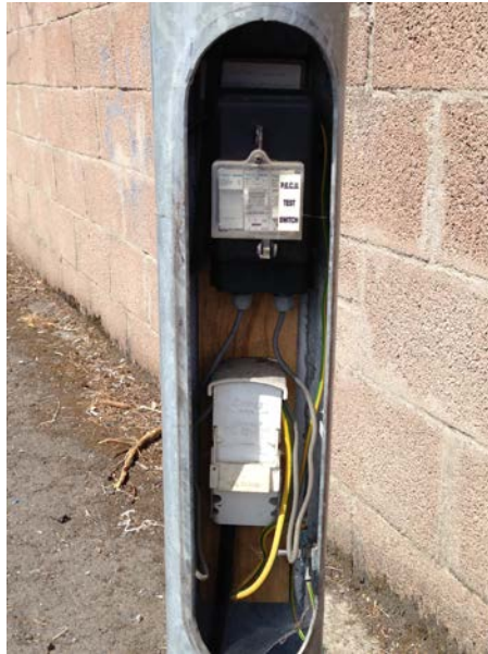
Example of Exposed Electrical Elements
