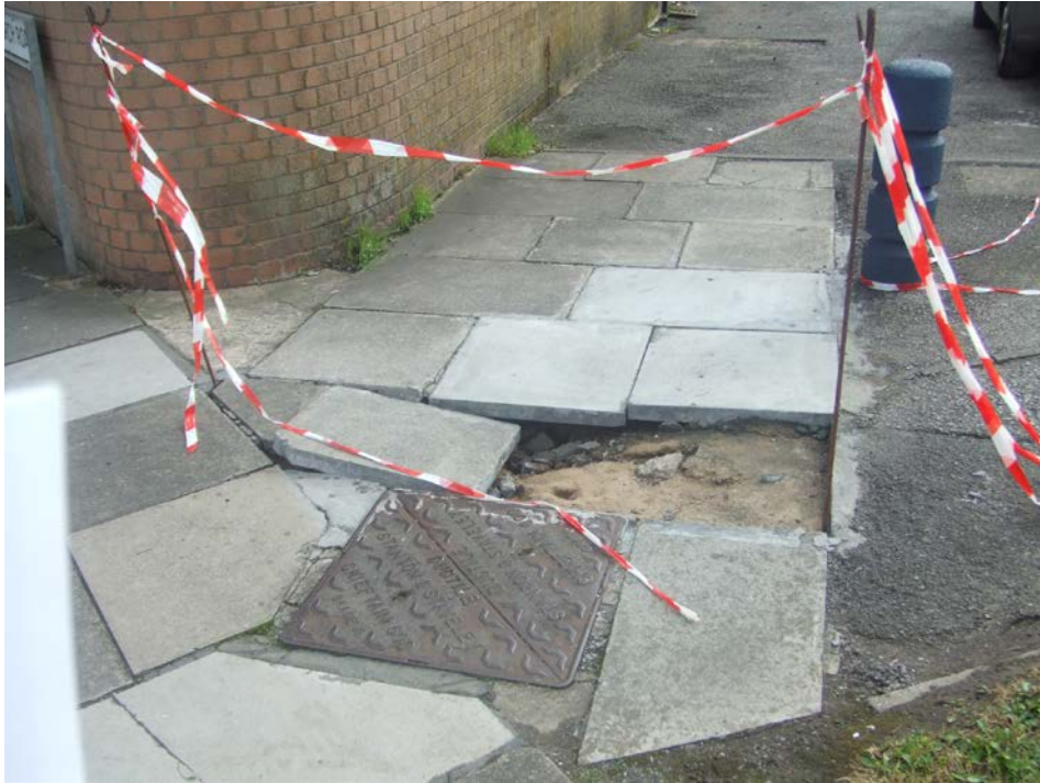
Example of Paving Defect
