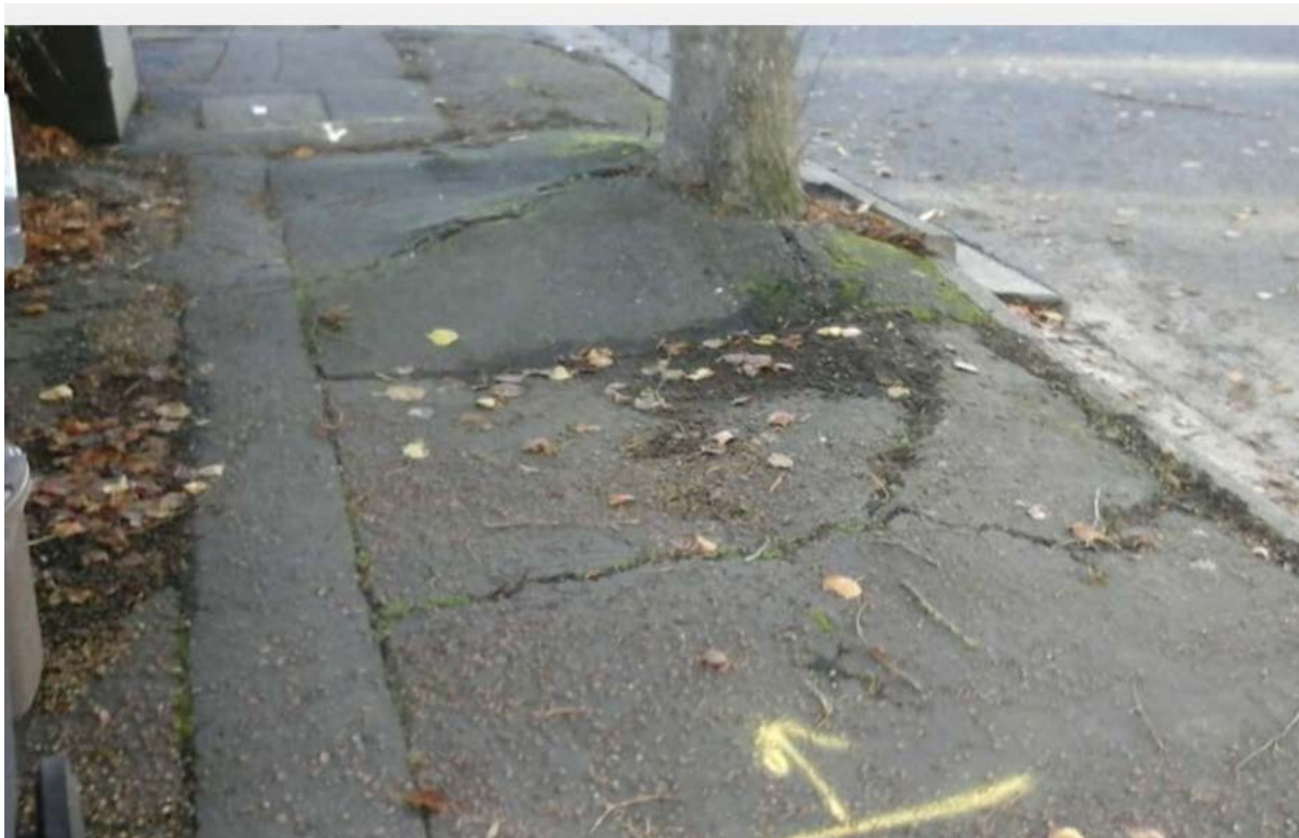
Example of Tree Root Damage
