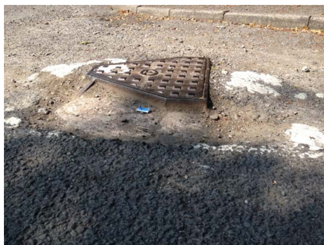
Example of Deterioration Around Ironwork
