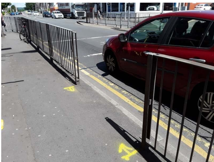
Missing Pedestrian Barrier
