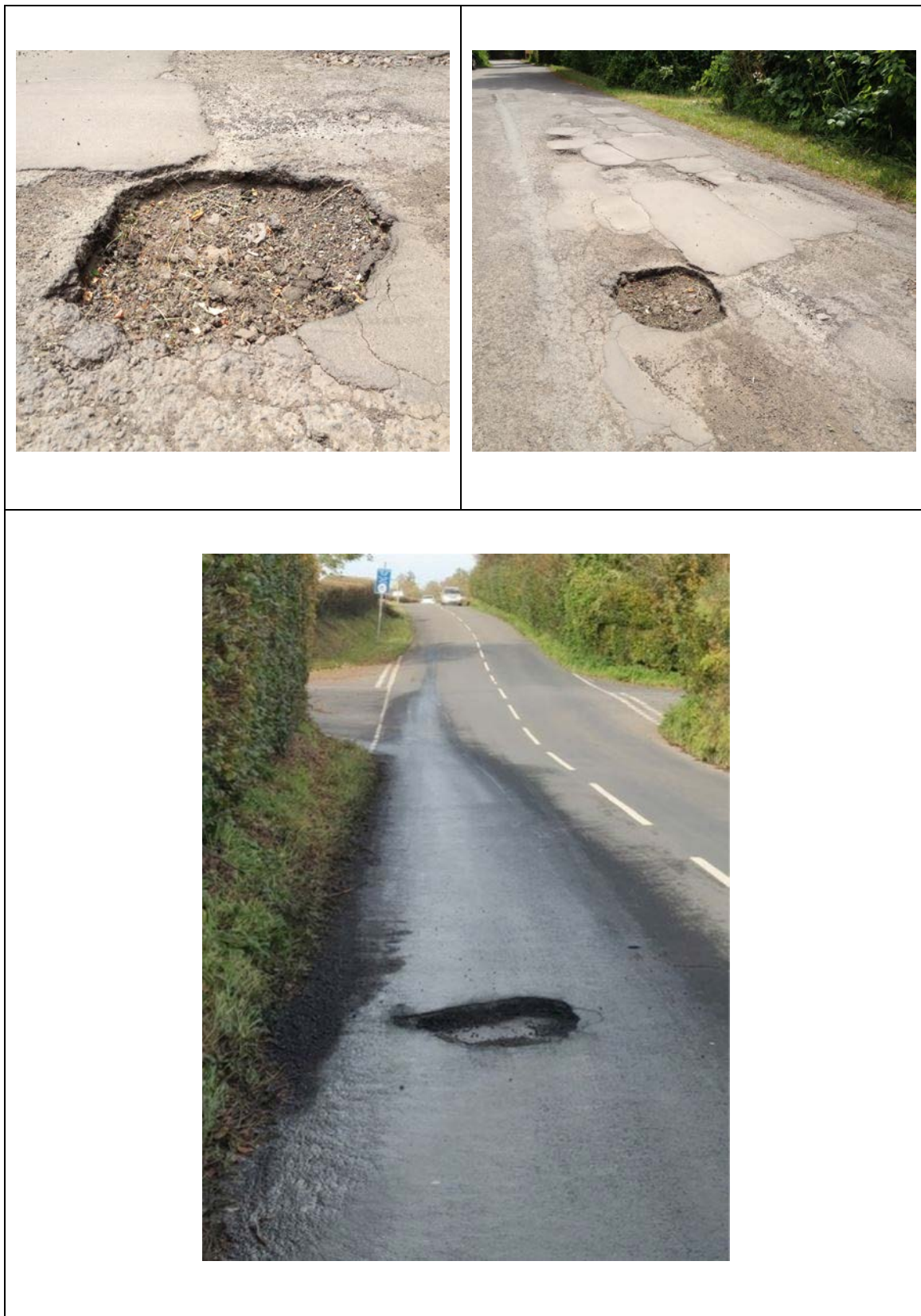
Examples of Potholes
