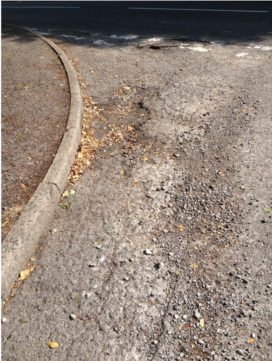
Example of Localised Surfacing Deterioration
