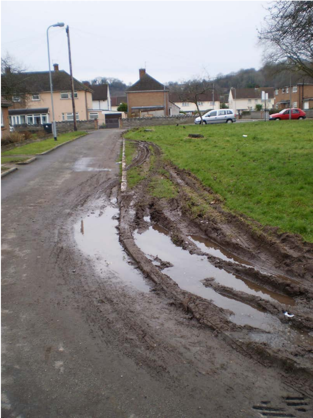
Example of Verge Defect
